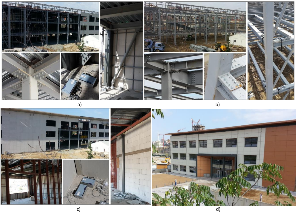
Figure 3. The building at the a) 1st stage: before the completion of slabs; b) 2nd stage: after the completion of slabs; c) 3rd stage: completion of the partition walls; d) 4th stage: completion of the construction. (Self-Elaboration).
