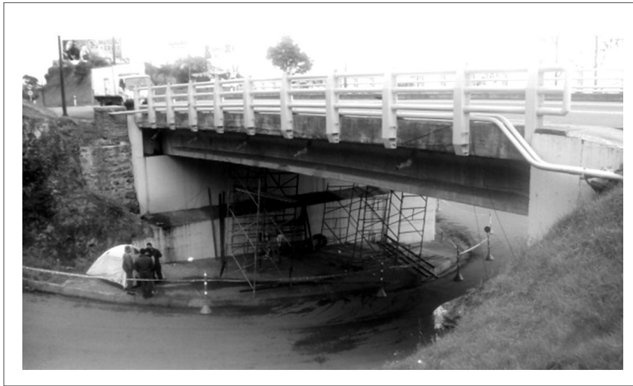
Figura 3. Vista en perfil del puente Boquerón simplemente apoyado de viga postensada y losa en concreto reforzado Figure 3. Cross section view for Boquerón Bridge, which is simply supported by a post-tensioned beam and reinforced concrete slab
