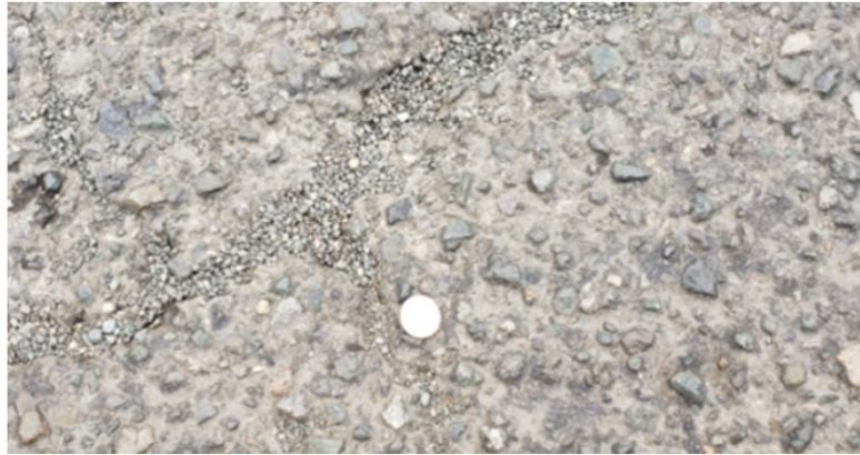
Figure 13. Surface damage for CDD=154.593 °C-days
