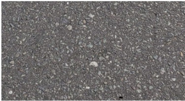
Figure 8. Surface damage for CDD=23.761 °C-days
