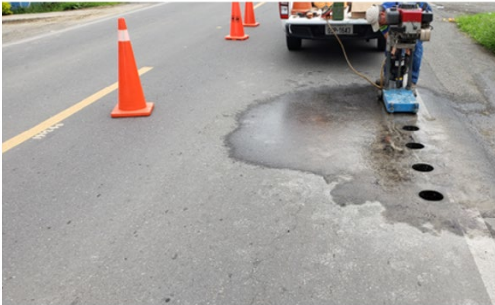
Figura 2. Core extraction in road Milagro- Naranjito- Bucay. Location 19+240
