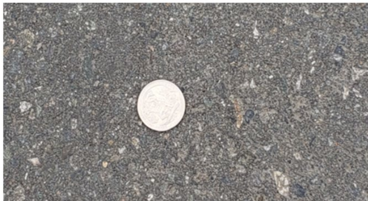
Figure 9. Surface damage for CDD=42.079 °C-days
