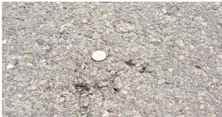
Figure 12. Surface damage for CDD=80.498 °C-days
