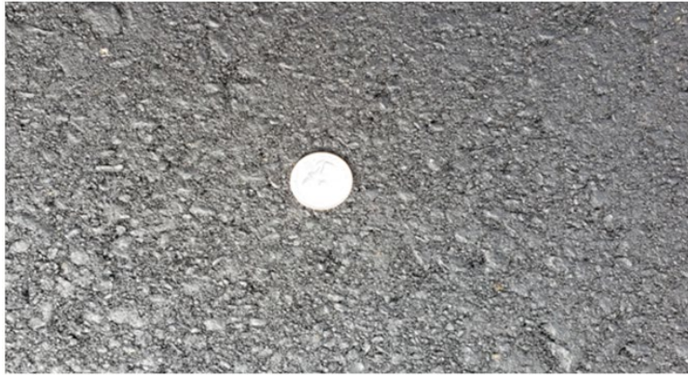
Figure 7. Surface damage for CDD=0 °C-days
